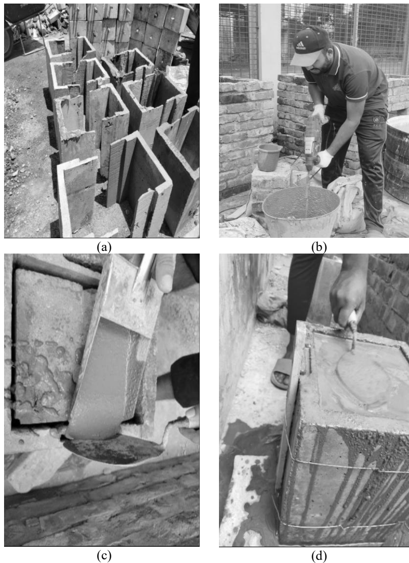
Figure 3: Installation of Jacket: (a) Precast jacket; (b) Grout mixing; (c) Grout filling; (d) Jacketed specimen.
