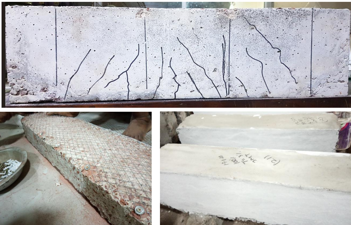
Figure 2: Damaged RC beam and preparation of ferrocement-retrofitting RC beams.
