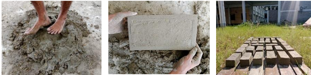
Figure 1: Preparation of the brick sample and prepared bricks placed for sun drying
