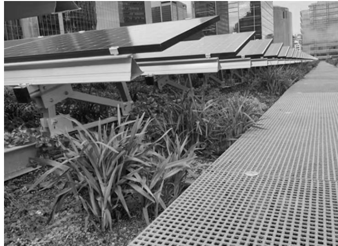
Figure 11: Rooftop view looking south, showing plantings around and underneath solar panels.
