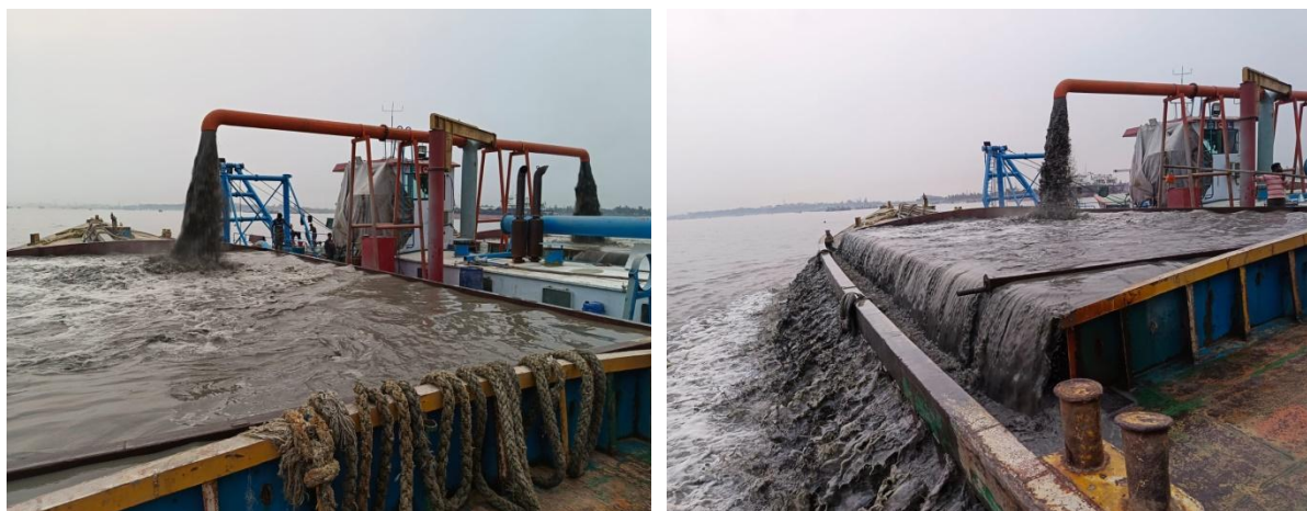
(a) Dredged material filling the barge (b) Spilling of mud-mix water into the river
