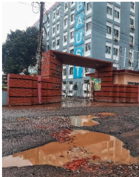
Figure 2: Illustration of a distressed pavement in front of the BAUST Campus
