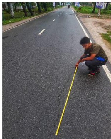
Figure 7: Low severity longitudinal crack
