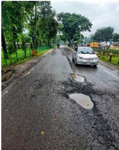
Figure 3: Pothole in the vicinity of a speed breaker
