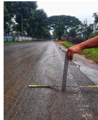
Figure 8: Medium severity rutting
