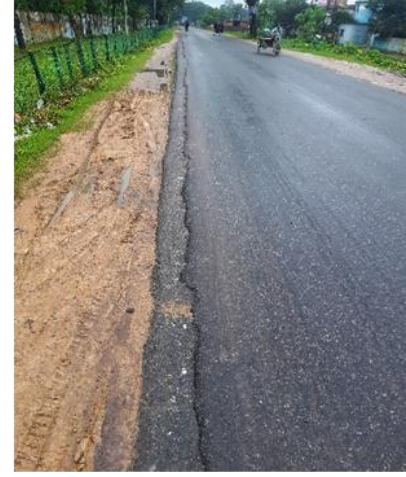
Figure 5: High severity edge failure
