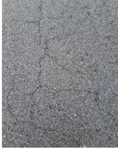
Figure 4: Medium severity alligator cracking
