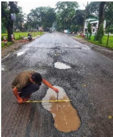
Figure 6: High severity pothole
