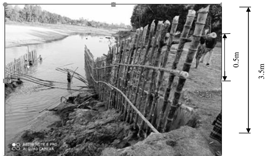
Figure 2.4: Construction of bamboo bandal structures in the right bank of Alaikhal River
