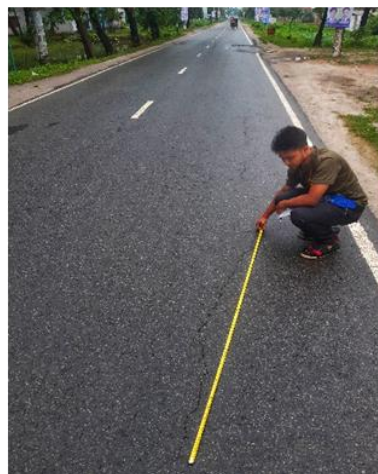
Figure 7: Low severity longitudinal crack
