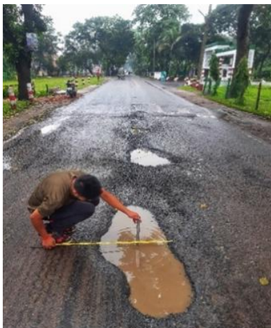
Figure 6: High severity pothole
