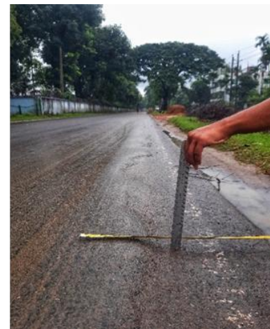
Figure 8: Medium severity rutting
