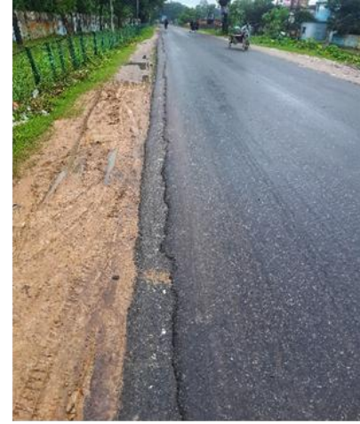
Figure 5: High severity edge failure
