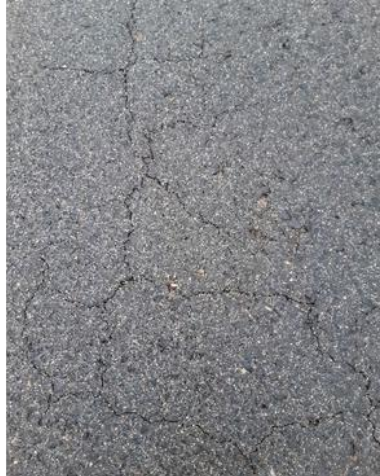
Figure 4: Medium severity alligator cracking
